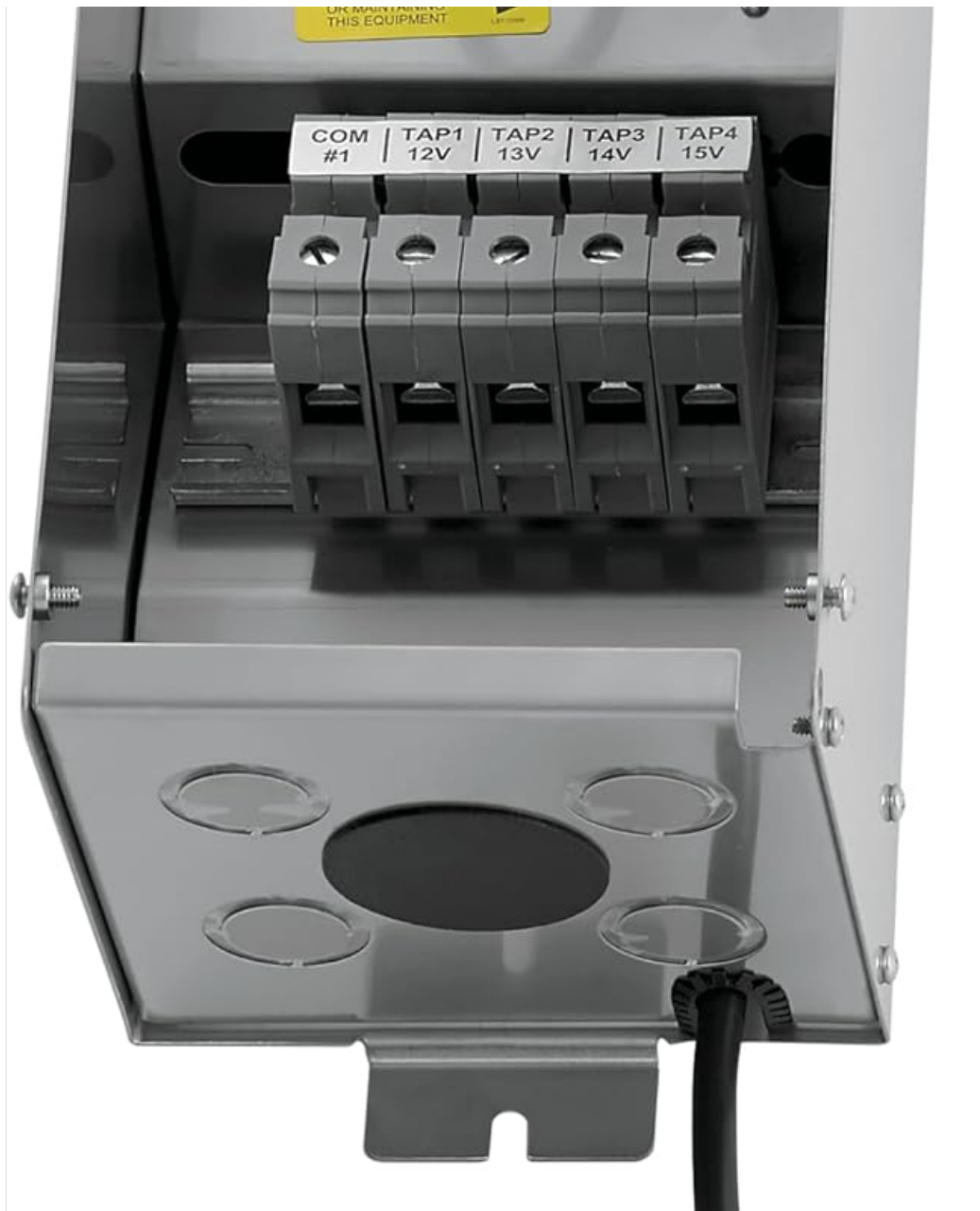
Figure 4.2: Close-up view of the tilted terminal board, showing connection points for various voltage taps (12V, 13V, 14V, 15V).
