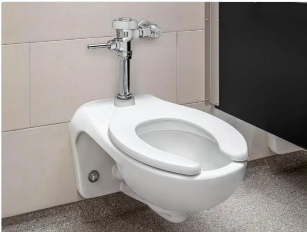
Image 2: Sloan Regal 180 Flushometer correctly installed on a urinal.
