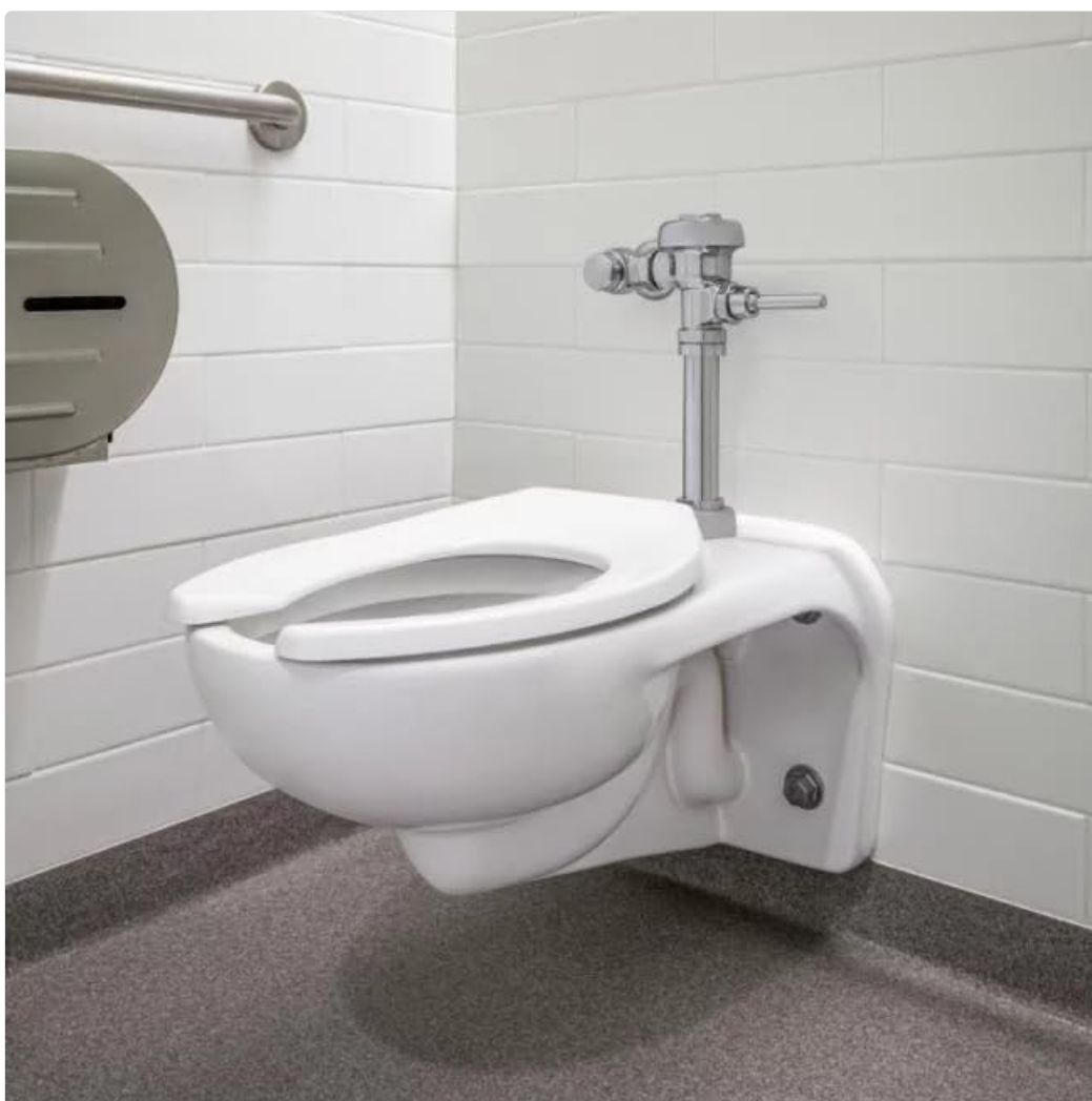
Image 3: Side view of the Sloan Regal 180 Flushometer installation.
