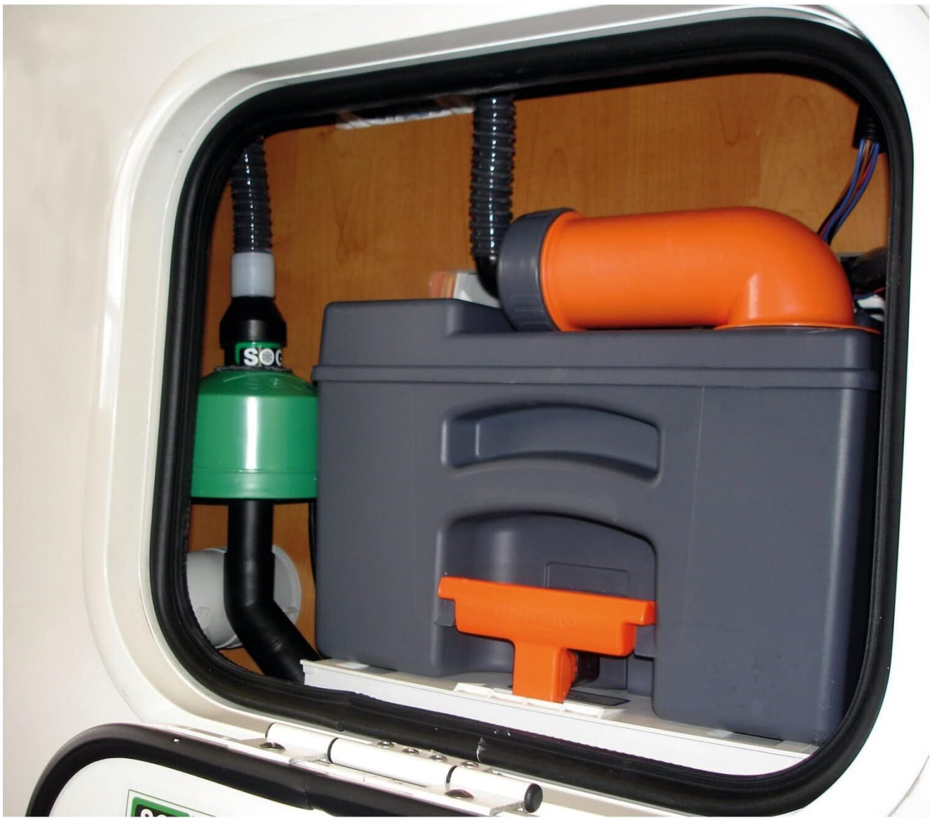
Figure 4: Installed SOG filter and fan unit within the compartment.
