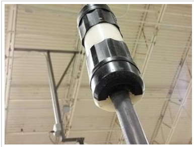
Figure 5.1: Detailed view of the internal wiring terminals. This image highlights the screw terminals where the electrical conductors are secured.
