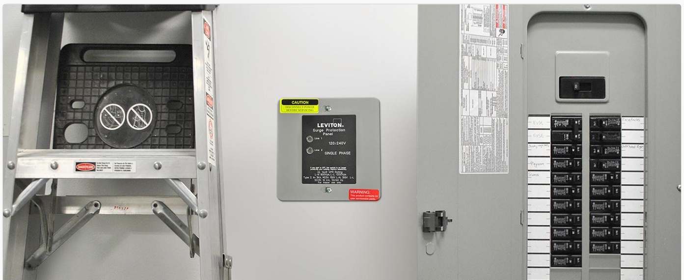
Image: An electrical service panel, illustrating the context of electrical installations. While the 8380-W is a point-of-use device, proper electrical system integrity is crucial for its effective operation.
