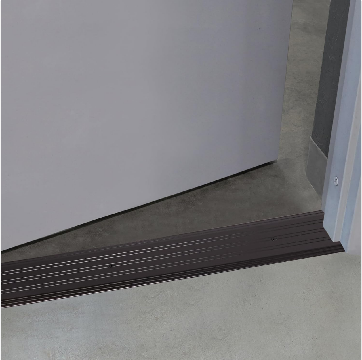
Figure 3: Example of the threshold installed at a doorway, providing a smooth transition.
