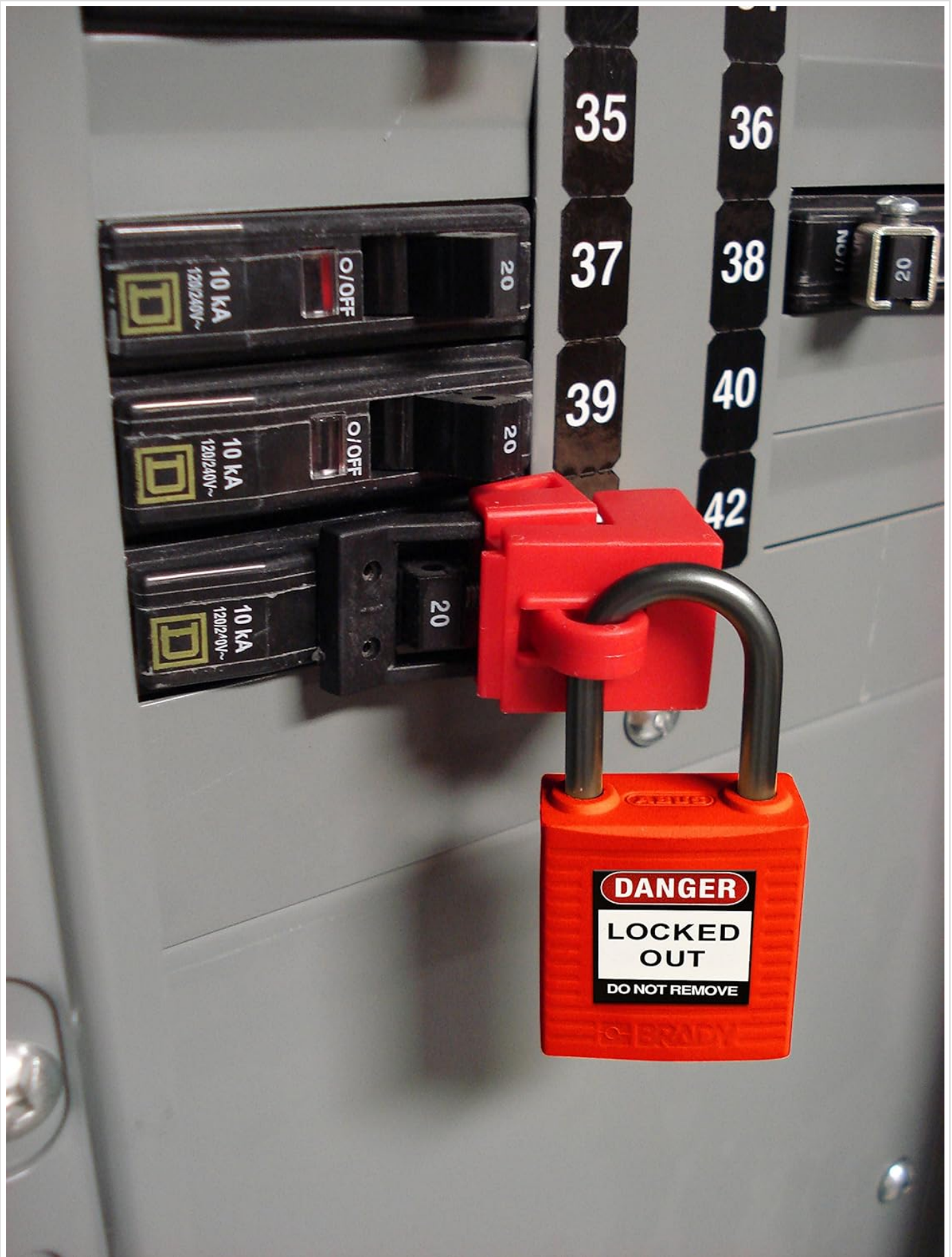
Image 2: The Brady Clamp-On Breaker Lockout securely installed on a circuit breaker, with a padlock and a "DANGER LOCKED OUT" tag attached.
