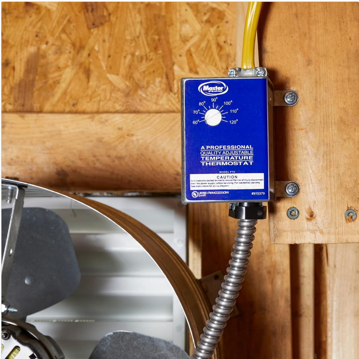
Figure 1: GAF Master Flow PT6 Thermostat installed next to an attic fan.
