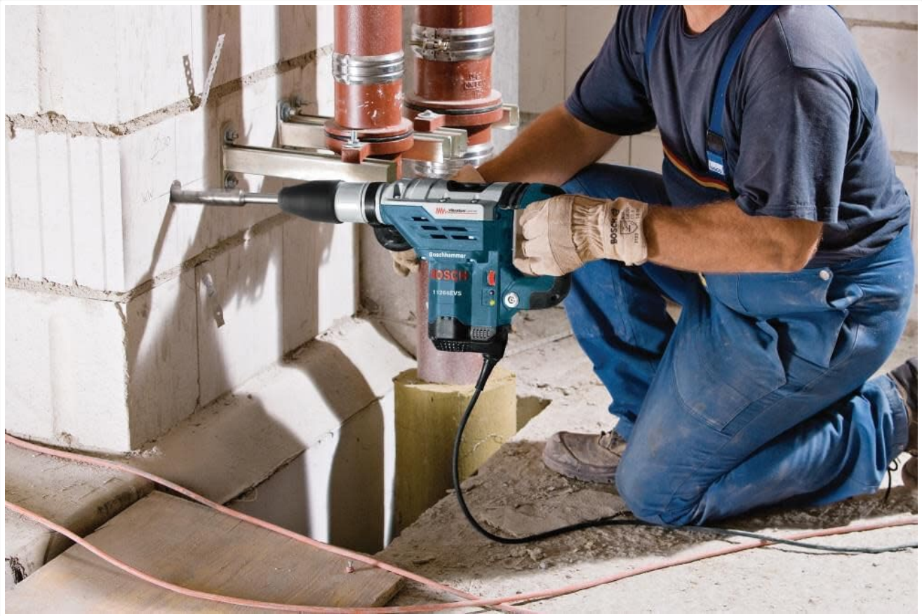
Image 5.2: A worker utilizing the BOSCH 11264EVS Combination Hammer for chiseling concrete on a floor, showcasing its use in hammer-only mode for demolition tasks.
