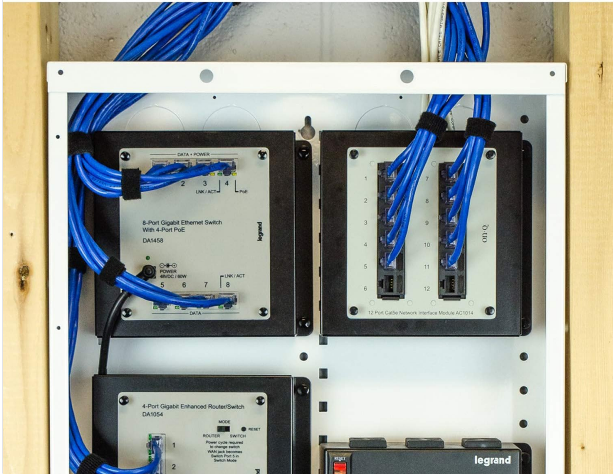
Figure 4.2: Components such as Ethernet switches and network interface modules neatly organized within the enclosure, with cables managed for optimal performance.
