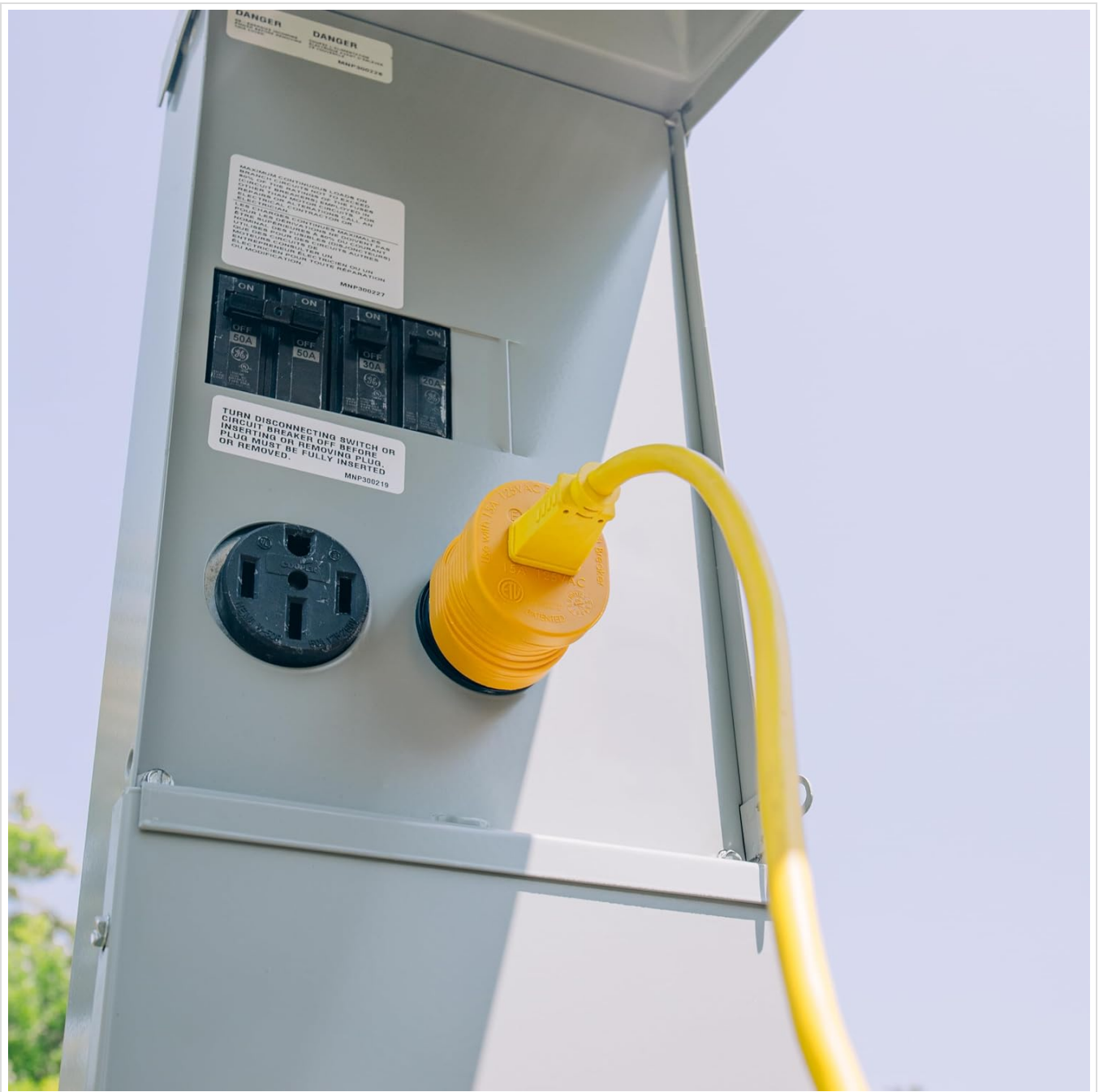
Image: The Camco PowerGrip adapter and RV cord fully connected to the power pedestal, ready for use.
