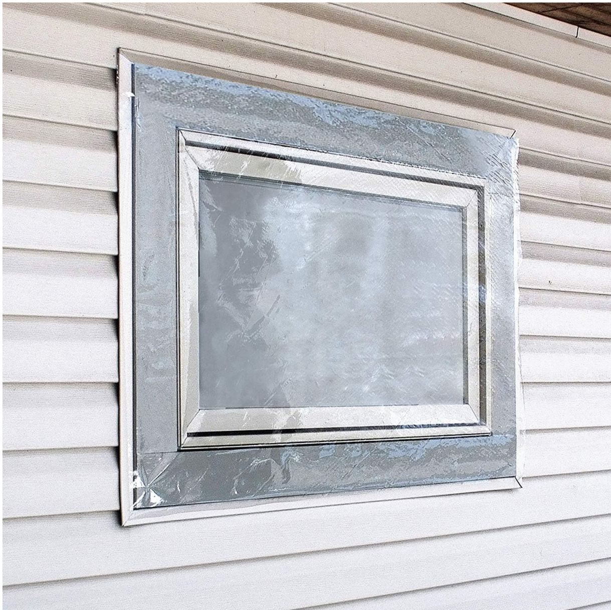
Image 3.1: Crystal clear vinyl sheeting applied to a window, demonstrating its transparency and use for insulation.
