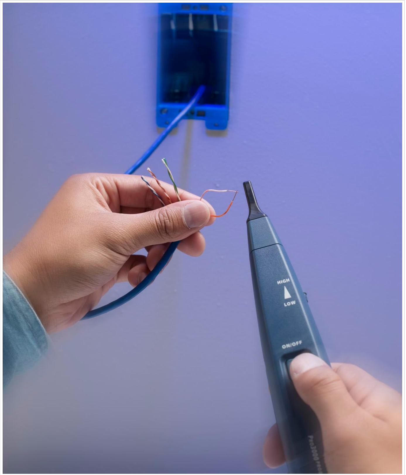
Figure 6.2: Demonstrates the Pro3000 Probe in action, tracing cables connected to a patch panel. The probe's tip is positioned near the cable connections to isolate the toned line.
