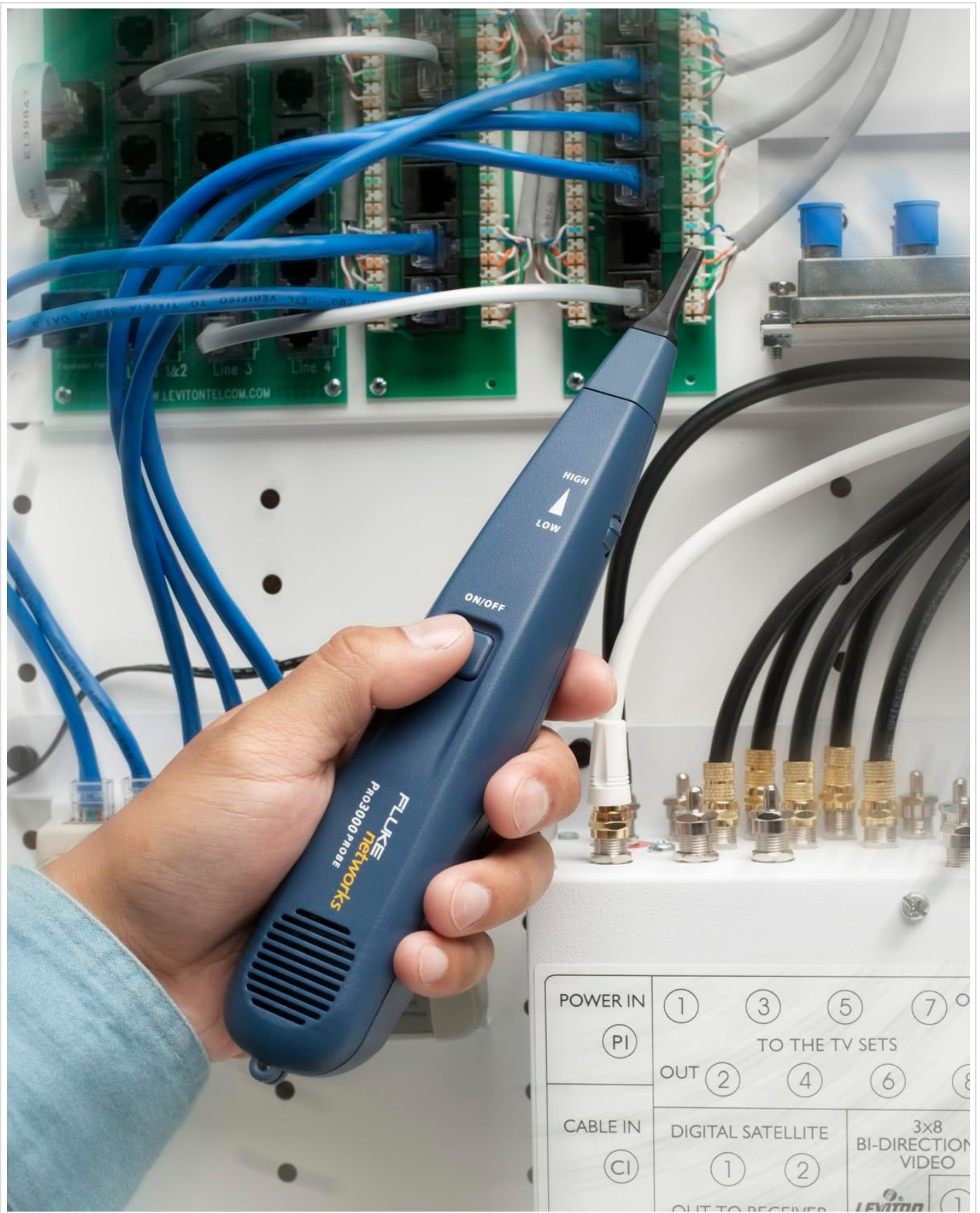
Figure 6.3: The Pro3000 Probe is shown tracing cables within a complex network cabinet, highlighting its utility in identifying specific lines among many.
