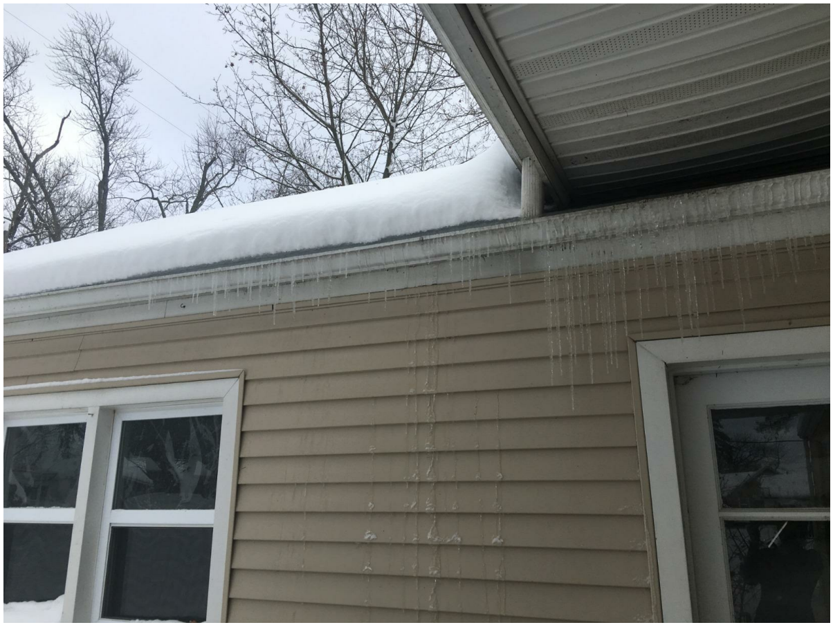
An example of the EasyHeat deicing cable installed within a gutter, demonstrating effective ice prevention with water visibly flowing through the downspout, even in cold conditions.
