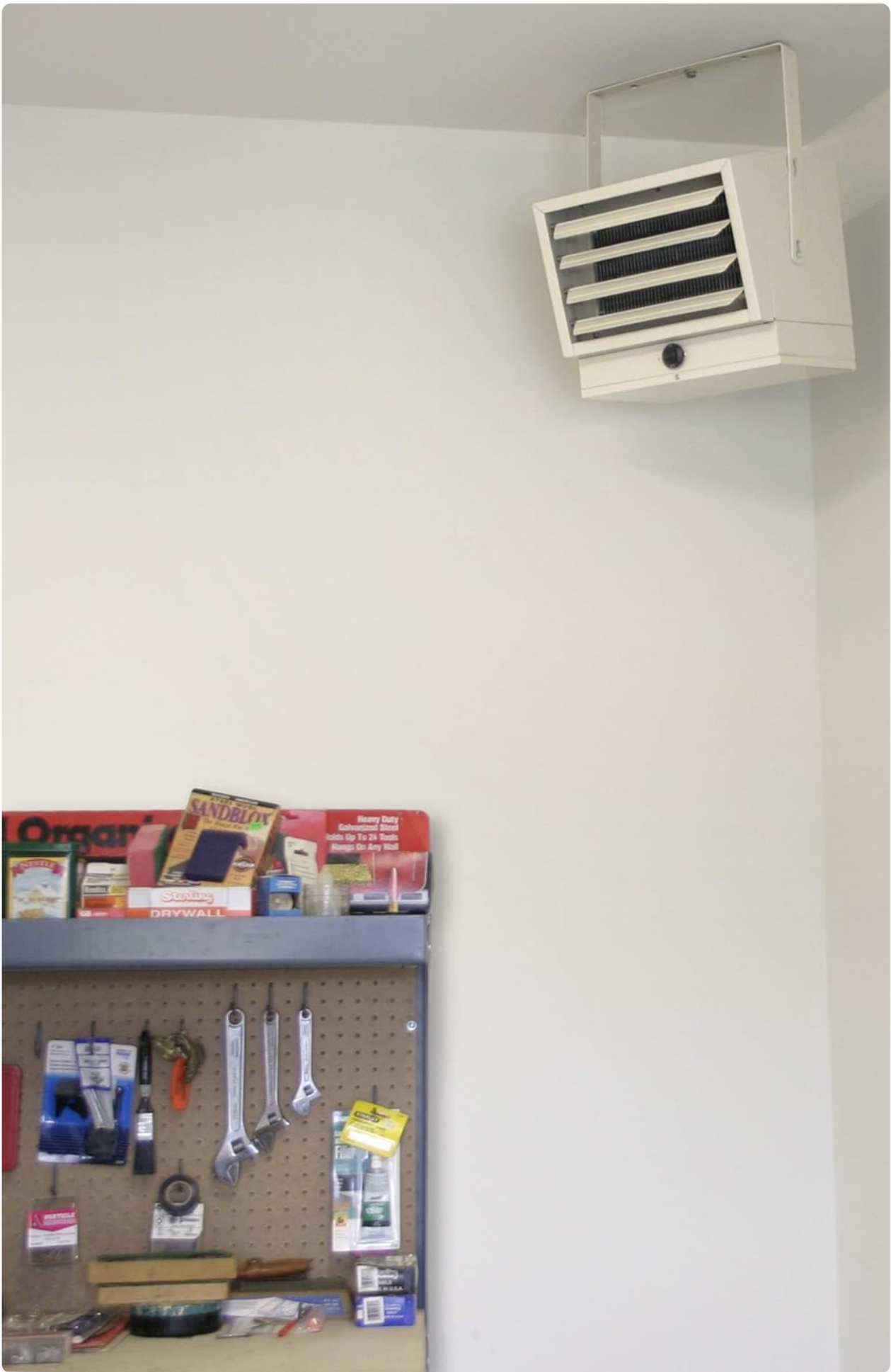
Figure 2: Fahrenheat FUH54 Electric Heater mounted on a ceiling in a workshop, angled downwards.
