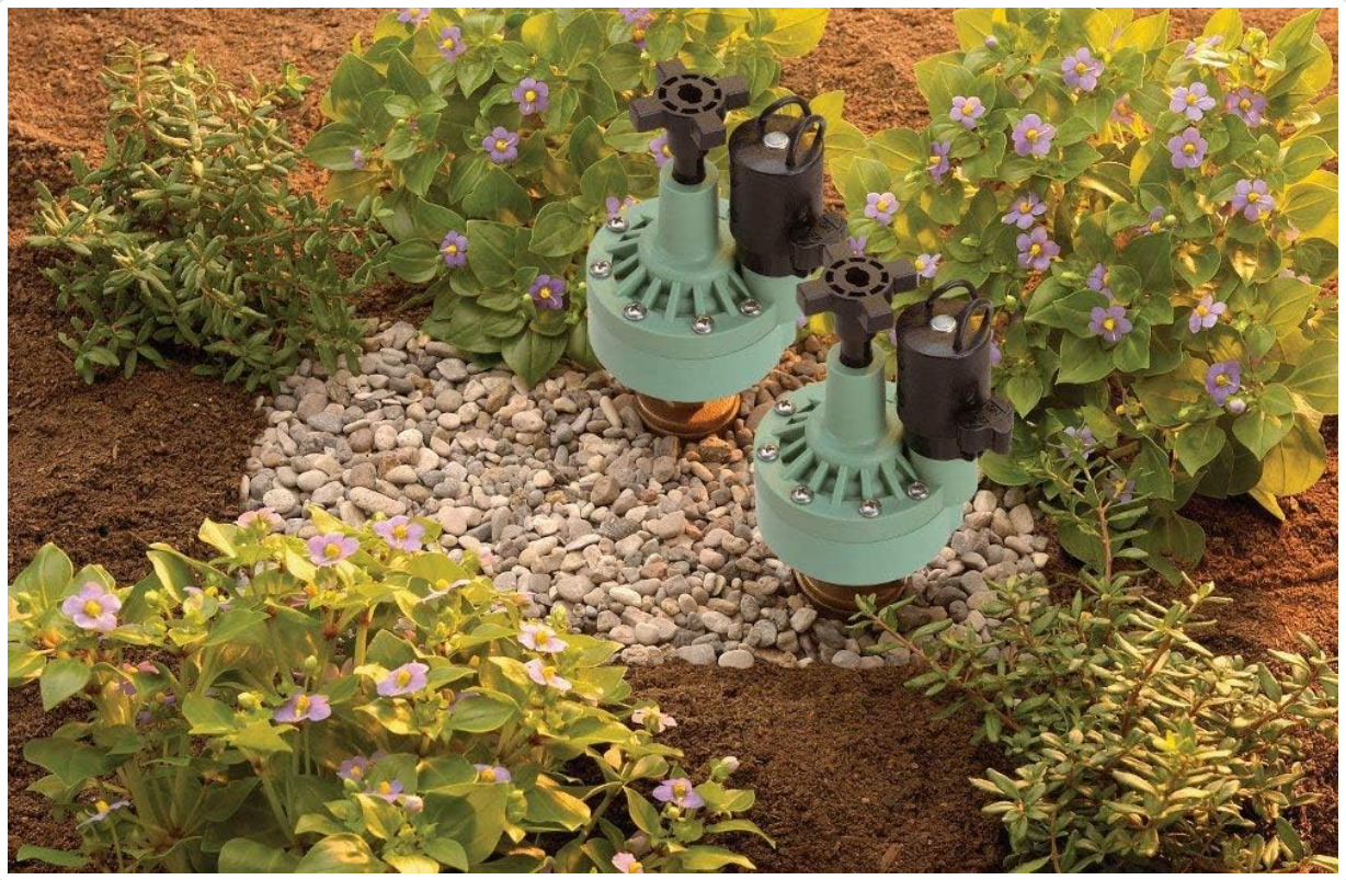
Image: Two Orbit 57029P automatic converter sprinkler valves installed side-by-side in a garden bed, surrounded by small rocks and plants, demonstrating a multi-zone setup.
